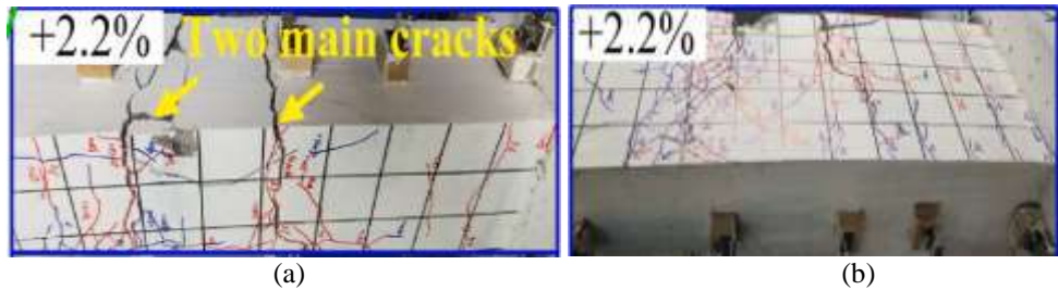
Figure 10: Cracking Formation of Experimental Beam RCB-KB5 by Qiang et al. (2019) (A) Top View of the Beam (B) Bottom View of the Beam
